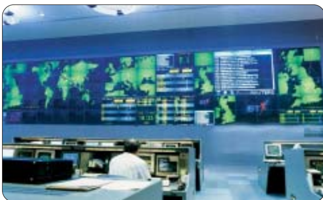
Telecomms Control Centre.
