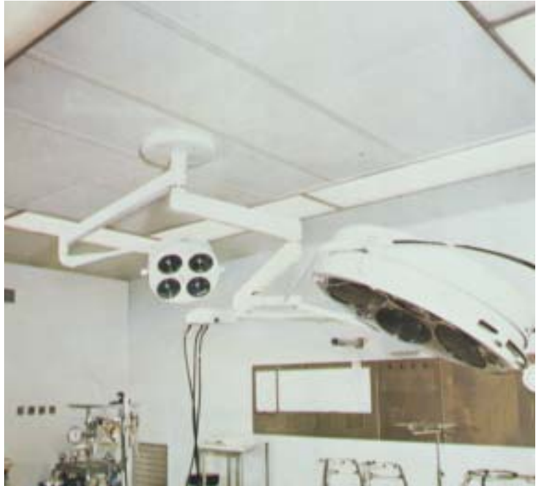
Typical installation of Laminar Flow Panels
